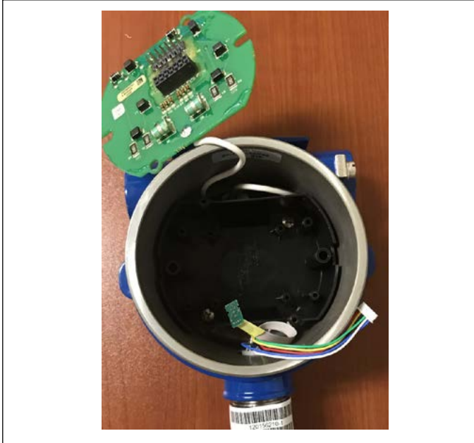
Fig. 13: Sensing Element disconnected
